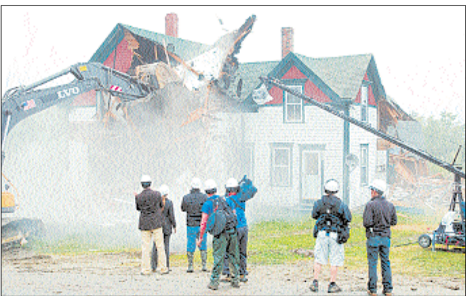
Members of the cast and crew of TV's "Extreme Makeover: Home Edition" watch and film the demolition of the Ray-Smith house in Milbridge on Tuesday.
